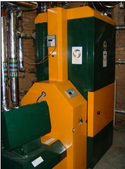
The 100 kW 'KWB' Boiler
