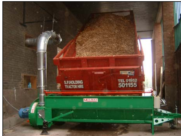
The first load of chips supplied by Midlands Wood Fuel. It takes about half an hour to unload the trailer. When not in use, the chip blower is swung out of the way to enable access to the service area under the Theatre.
