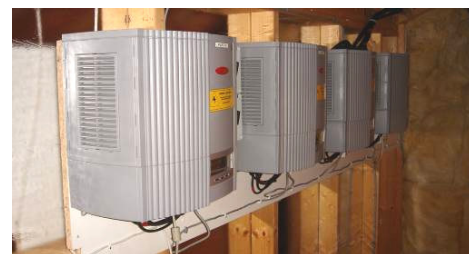
Four of the 10 inverters installed
