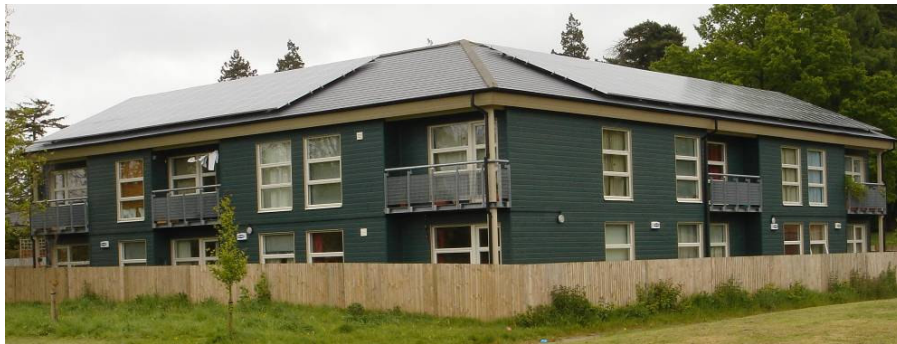
Kidby House showing both south and west facing arrays
