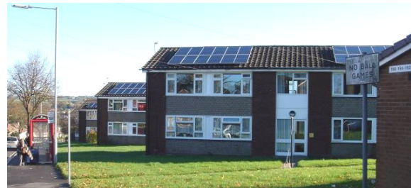
Photo showing systems installed on blocks of flats
