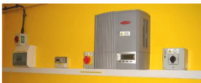
The PV electrical installation of one of the schools
