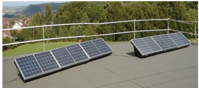
The array mounted on the flat roof
