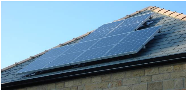
The array mounted on the pitched roof
