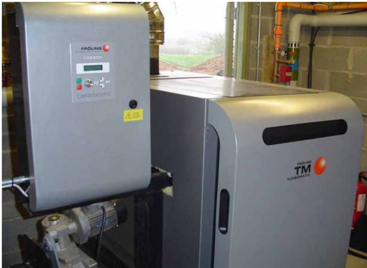
Fröling Turbomatic 55kW automatic woodchip boiler
